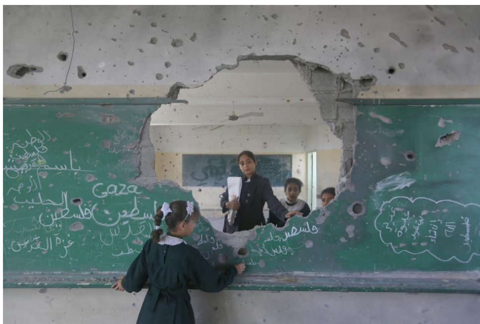
Eleven-year-old Manar and her friends at their school in Gaza, which was badly damaged during the 2014 conflict: 'The damage scares me. The classes are overcrowded and the water leaks in when it rains. But I love my school.' (2015) Photo: Iyad al Baba/Oxfam
